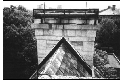
All chimneys should be kept, regardless of whether they're for functioning or non-functioning fireplaces.
