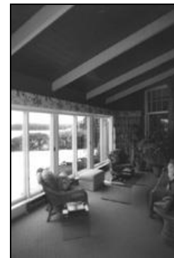
The sunroom is not insulated and considered to be sub-standard.
