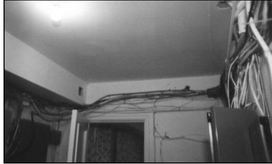
The house was rewired in the 1950s; it should be rewired again.
