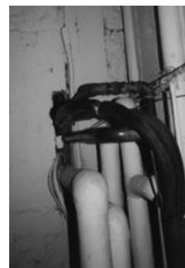
Asbestos and lead should as much as possible be removed
