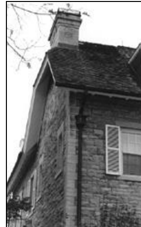
The eavestroughs and downpipes need to be replaced.
