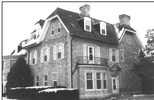
Windows in a building are major determinants of a building's character. They should be restored where deterioration has occurred.
