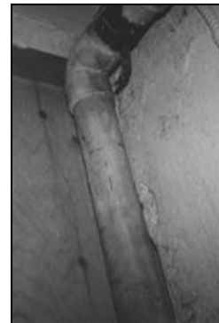
Galvanised waste piping beyond useful life.
