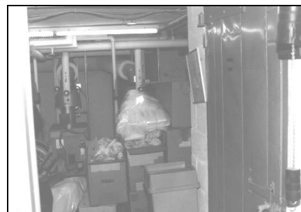
Egress routes through the basement are cluttered with hospitality storage.
