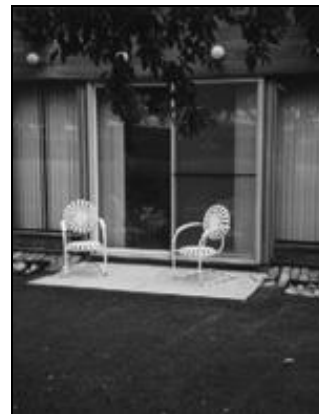
The patio on the north side of the pool building is functionally unusable.
