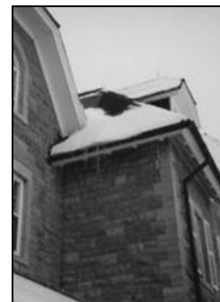
The exterior masonry needs to be repointed.
