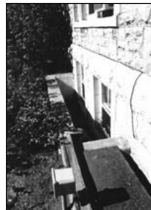
There is no evidence of existing perimeter drains to evacuate groundwater from the foundations.
