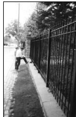
Front fence and gates are at end of useful life and need to be replaced.
