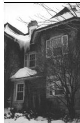
Insufficient insulation causes energy loss.
